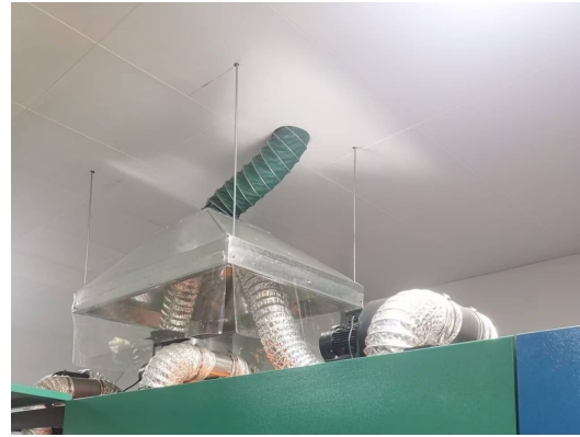
吹瓶机（拉吹机）上方集气罩+软帘
